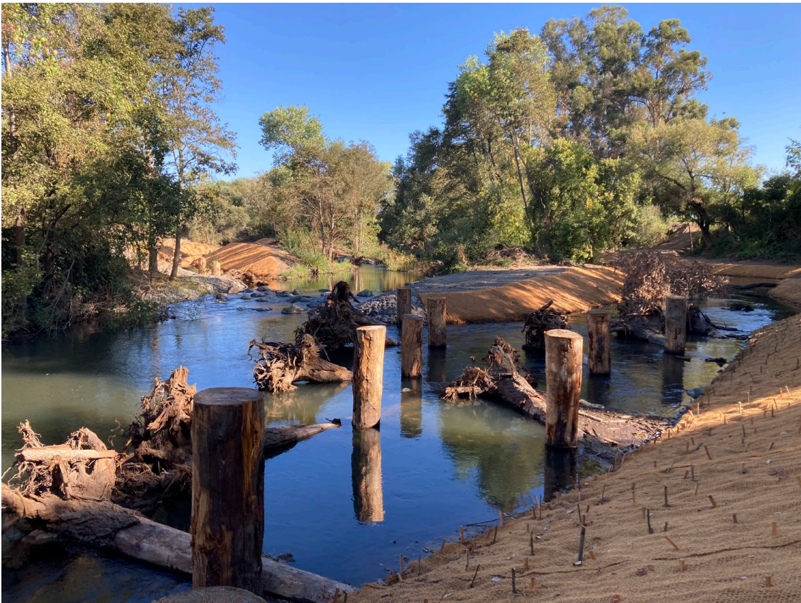
Reach 2 sites on September 4, 2024. View is looking back upstream with the main channel of Dry Creek in the center and a newly constructed side channel visible on the right and the outlet of a newly constructed side channel visible to the left of the main channel.
