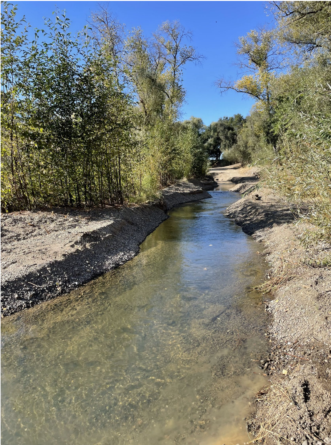
Photo of newly opened portion of the habitat channel. Photo is looking back upstream along the constructed habitat channel in Reach 5A. Photo taken October 9, 2024.
