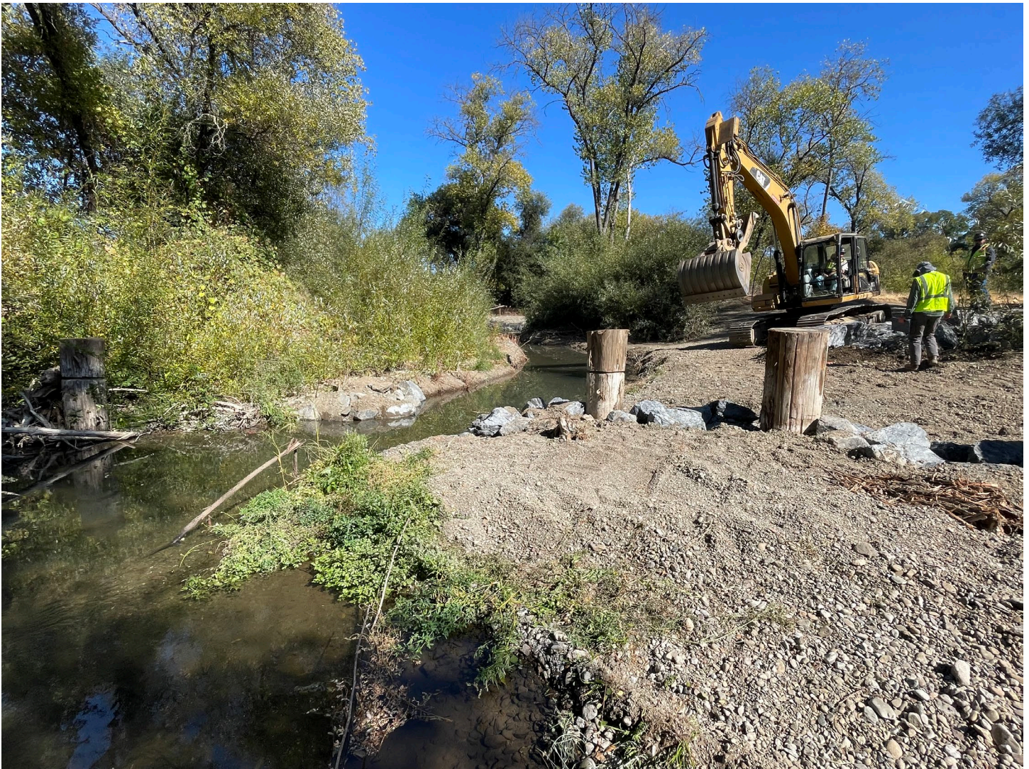
Photo of newly opened portion of the habitat channel. Photo is showing the inlet connection from Dry Creek into the habitat channel in Reach 5A. Photo taken October 3, 2024.
