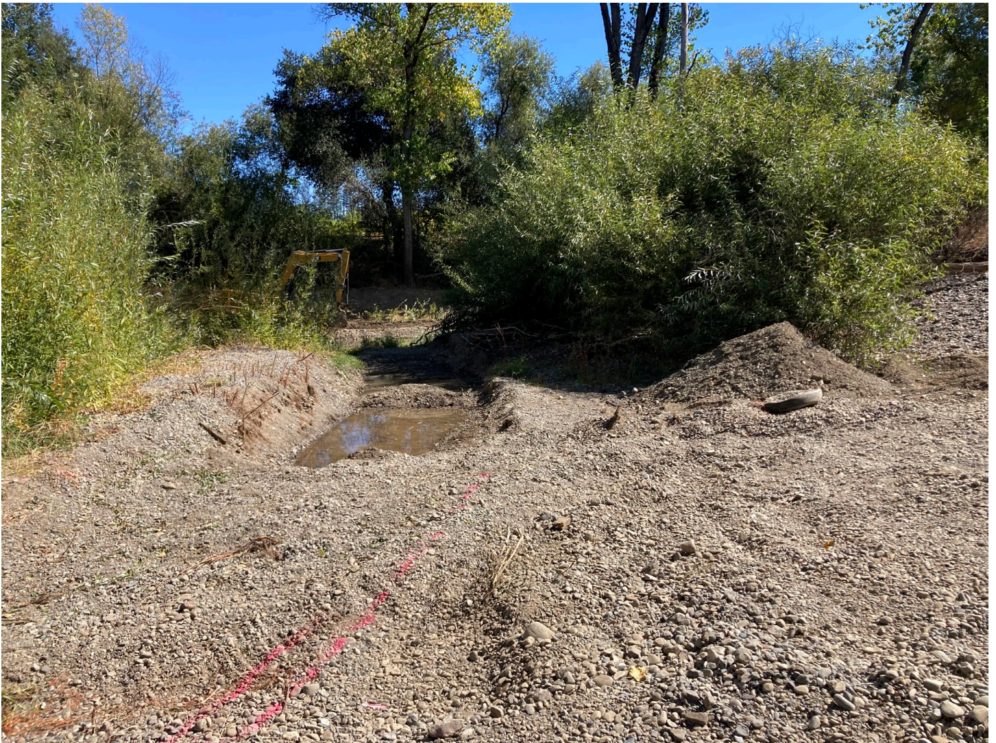
Photo showing portion of the Reach 5A Channel that had filled in. Habitat channel shown is in process of being re-excavated. Photo taken September 26, 2024.
